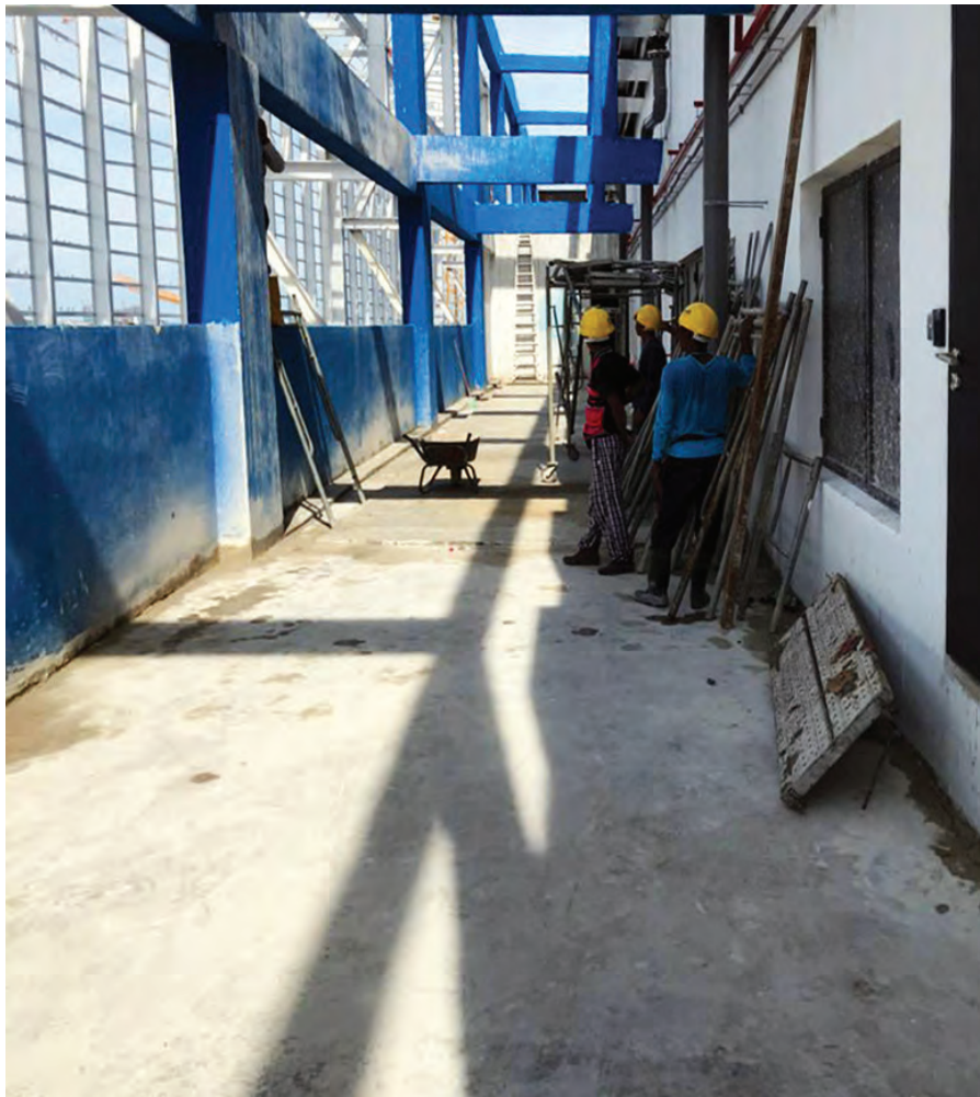
A number of areas in the theatre needed to be waterproofed, such as flat surfaces, lift shafts, bearing walls, pump room, storage tanks, balconies, corridors, bathrooms and kitchens, as well as some sections of the stage.
