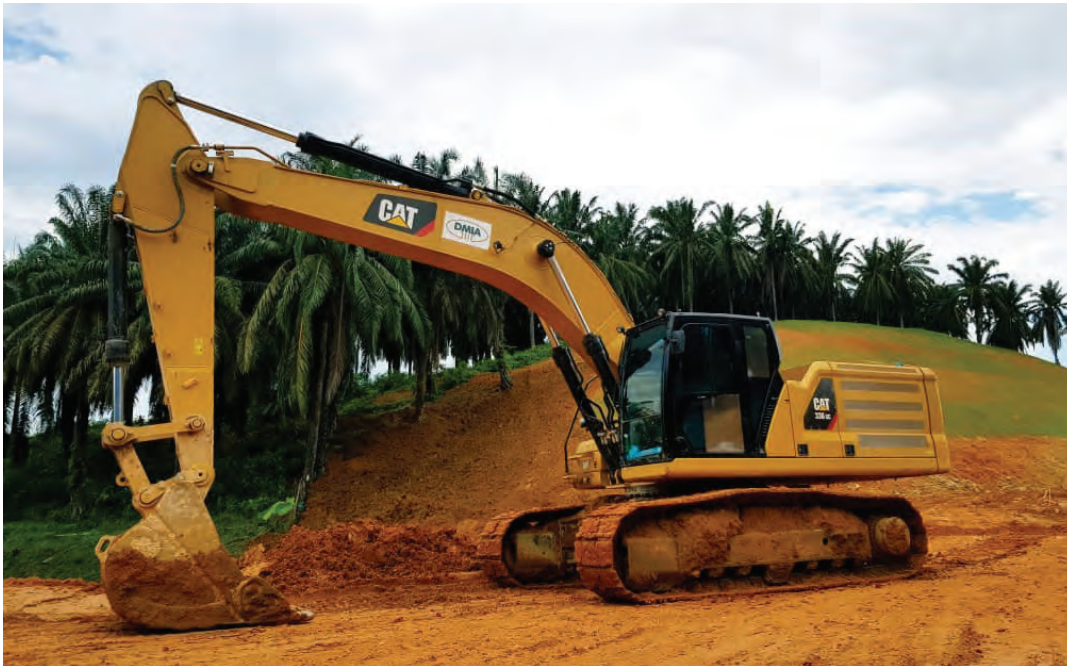
Sime Darby Industrial has supplied various machines to Dhaya Maju Infrastructure (Asia) Sdn Bhd - including Cat machines - for use in the West Coast Expressway project in Malaysia.
