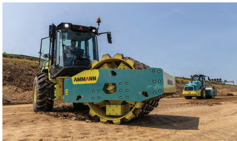
Ammann’s ARS 200 HX smooth drum roller and ARS 220 HX padfoot drum roller are both involved in the project during compaction work. The machines are equipped with innovative technologies, such as the ACE force and Q Point telematics systems, thus delivering better performance on the job site.
