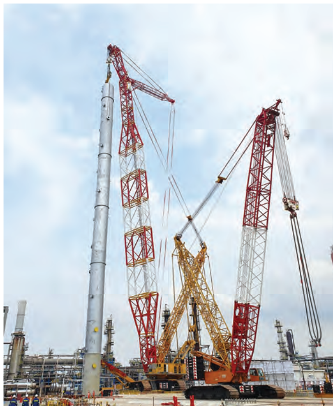
The Demag CC 8800-1 crawler crane with the boom booster kit is seen here lifting the 510-t splitter tower, working in tandem with a smaller Demag model, the CC 2800-1.
